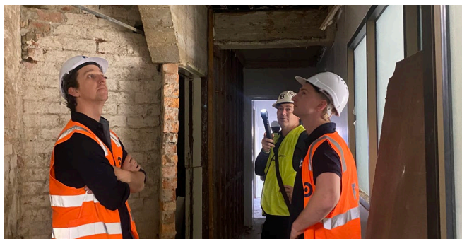
Construction work is underway at the Ballarat Foundation Giving Hub in Lydiard St.
